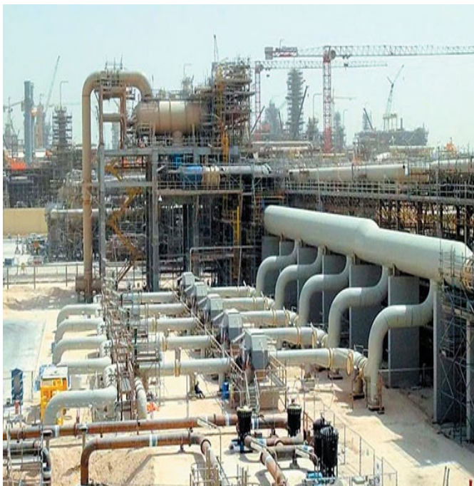
Gas Inlet and Process area - Barzan Onshore Project ▲
